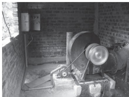
Figure 3 The low-head turbine at Magdalena drives an induction motor as generator (IMAG) with controller (photo: Robert Simpson)
